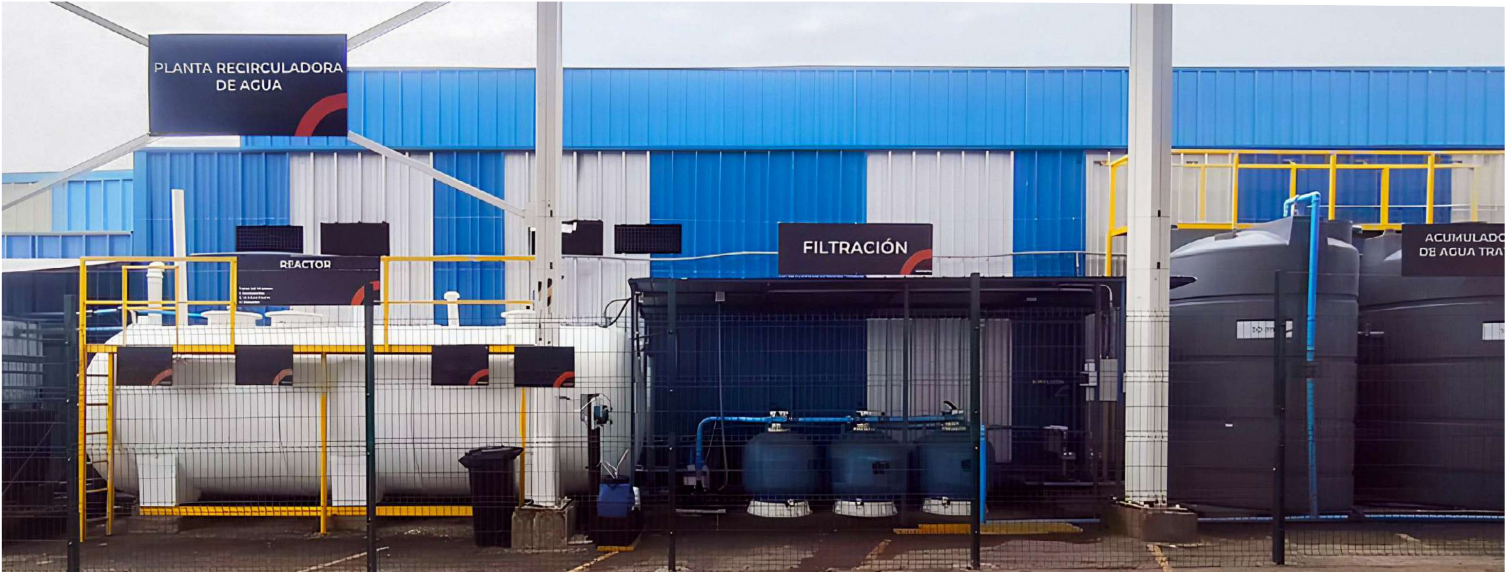
Water recycling facility at Astara Chile
